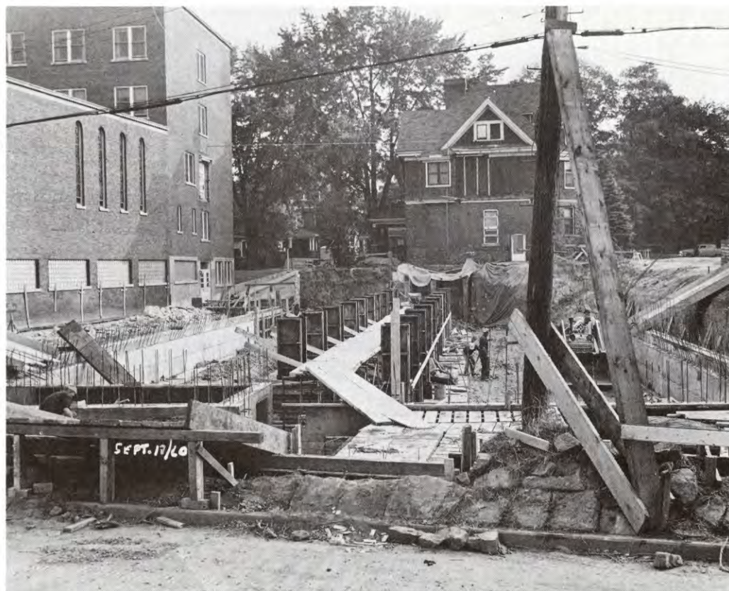
Photograph taken from Yates Street behind the Sisters' Residence at 151 Ontario Street showing the construction of the new wing. W.E. Shore photo.
