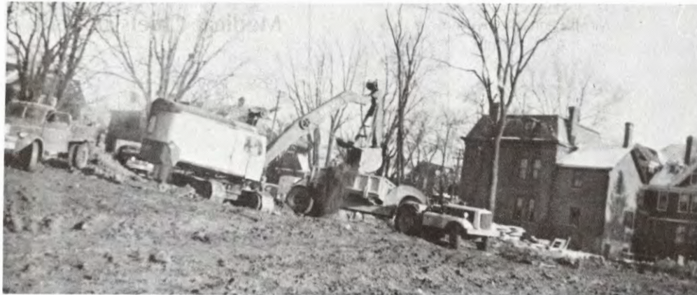
The excavation for the Hotel Dieu Hospital on the Conroy property in 1950 after the Leonard St. John apartments were demolished. The Dawson house is seen in the background.
