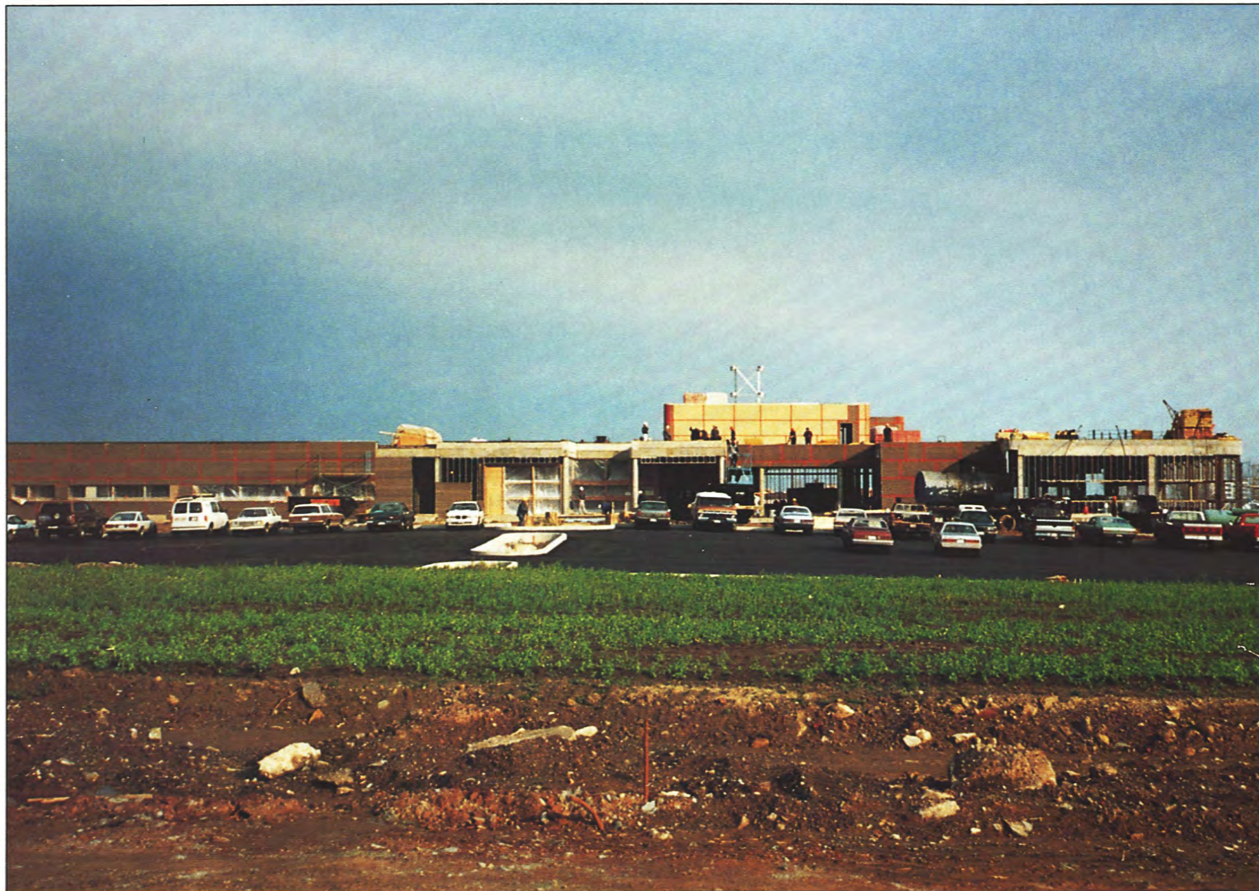
The exterior of St. Joseph's Community Health Centre nears completion of construction in the autumn of 1989.
