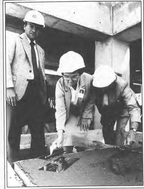
Sister Joan O'Sullivan (centre) puts a finishing touch on the west wing construction with John Shea (right), Chairman, Board of Trustees.
