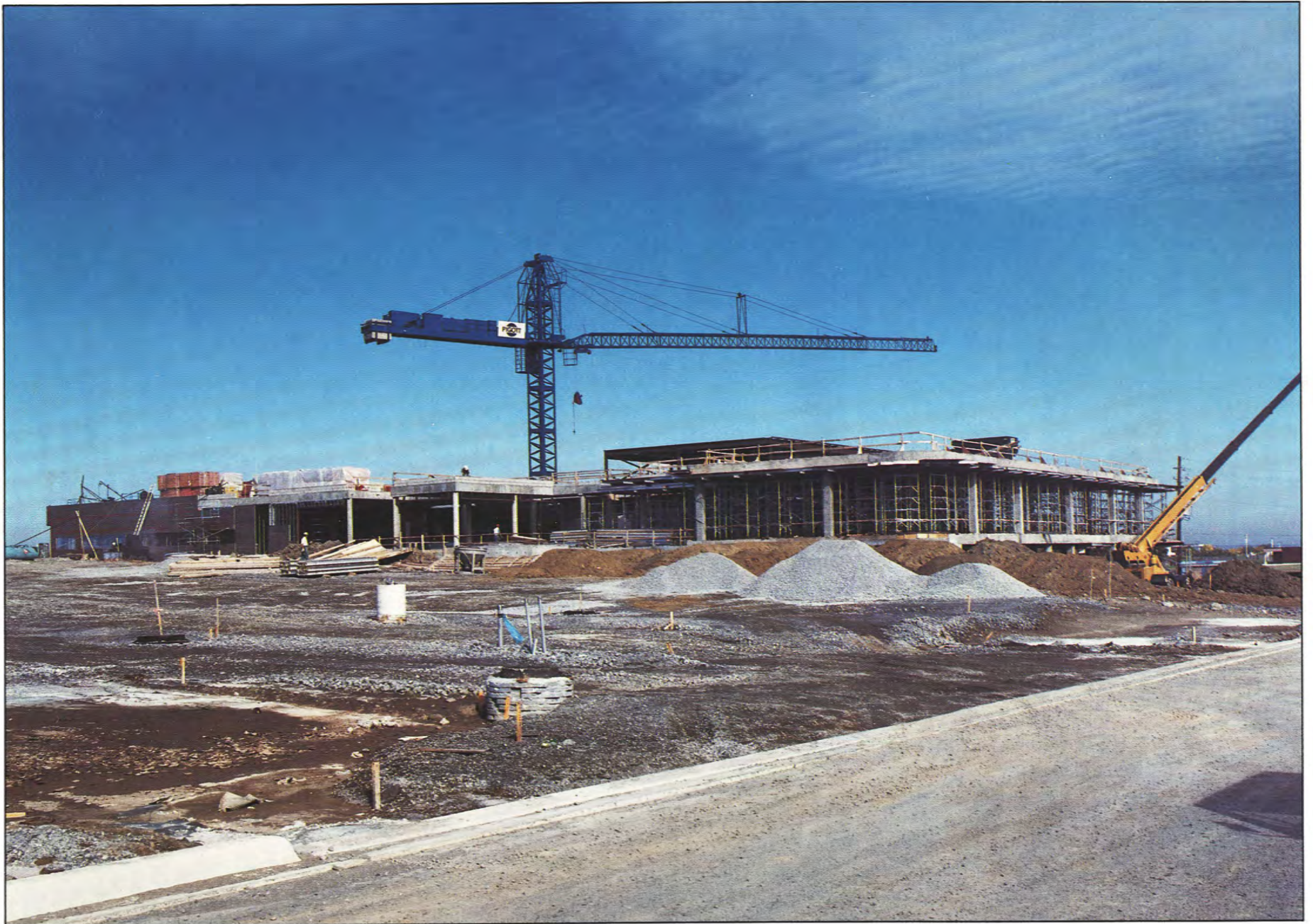
St. Joseph's Community Health Centre at King Street East and Nash Road under construction in 1989. By the end of the 1990s, it will serve a population of 109,000.
