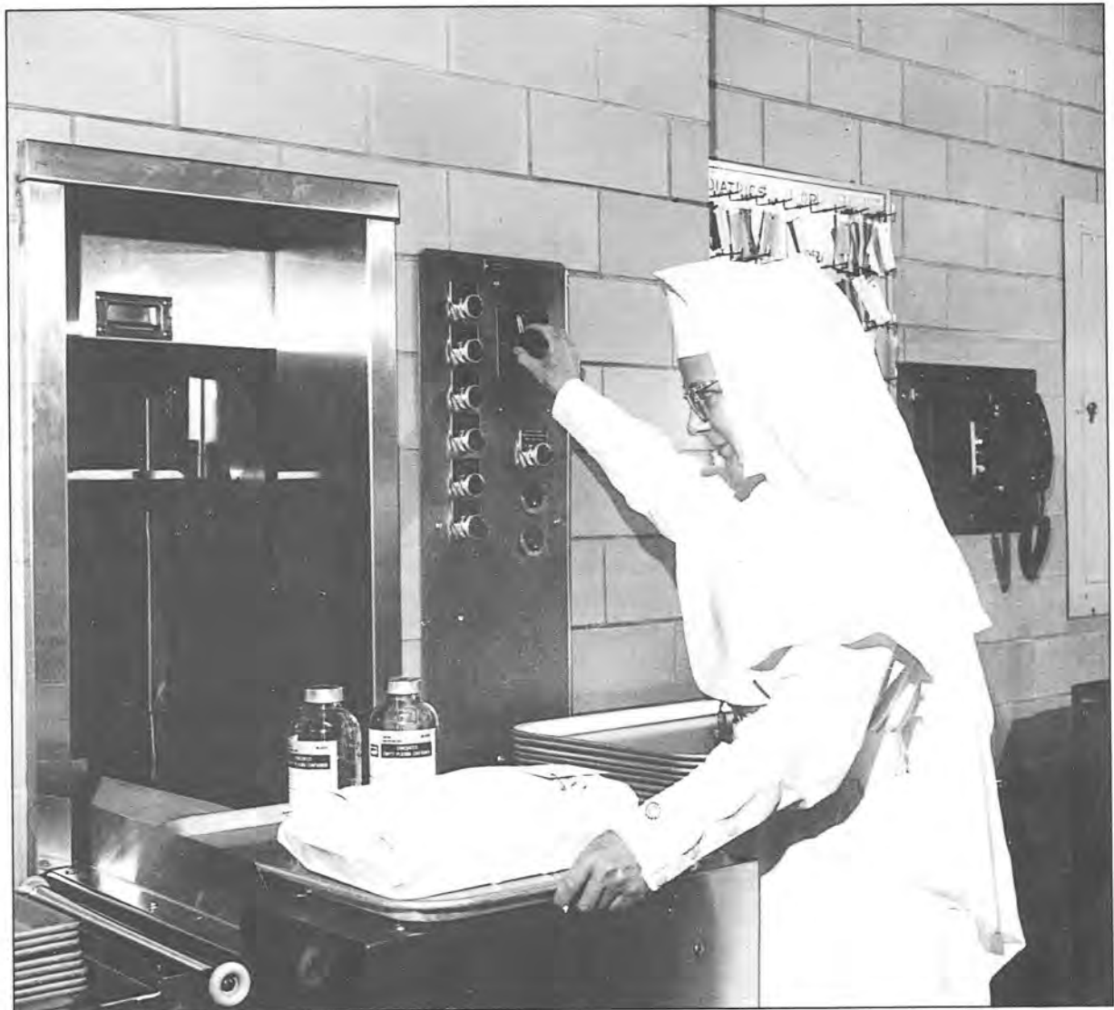
The Friesen concept at work: Sister Mary Rose Pautler pushes the button for the floor designated to receive items from the trayveyor.
