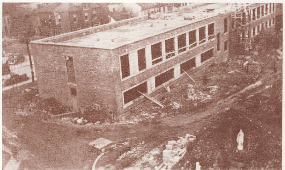
The Jeanne Mance Nurses' Residence under construction on Brock St. Four stories were added later. Grotto was still in garden.
